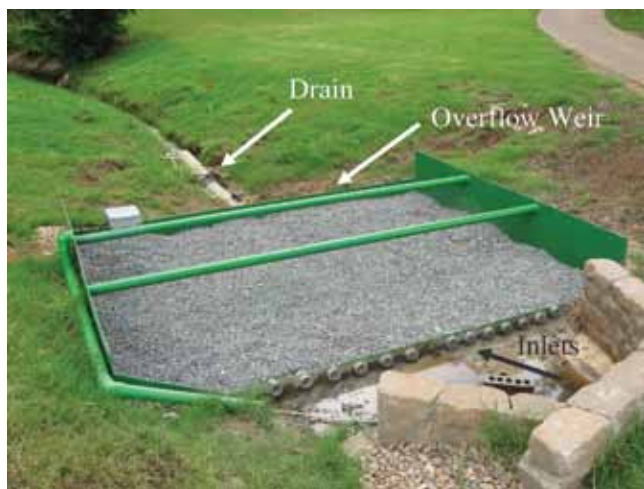
Fig. 1. Picture of the phosphorus (P) removal structure with runoff inlets, drain for treated water, and overflow weir. The P sorption material in the structure is 2712 kg of 6.3- to 11-mm-diameter steel slag.
